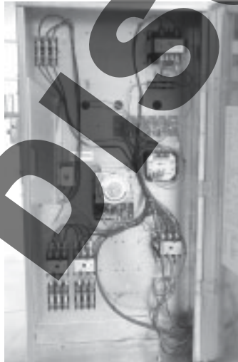
Large Electrical Panel
