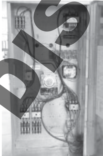
Large Electrical Panel
